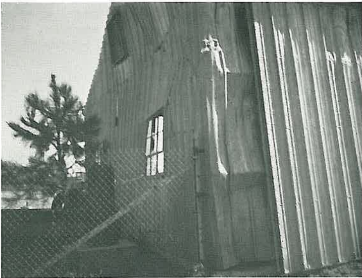
The south side was most heavily damaged. Note holes where objects were blown through the building. Doors were moved from the other side of the building and wire nailed over holes to prevent looting.
